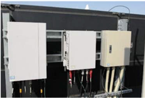
Figure 3. Base stations and antennas for rooftop installation (Source: UQ)
