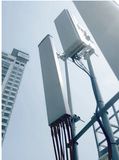
Figure 4: Co-located 32T32R and 8T8R MIMO antennas
